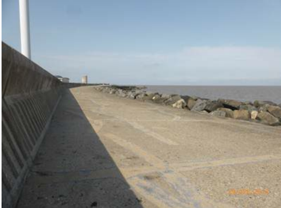
Figure 8.5: Lowestoft Ness-Hamilton – coastal dike. In the example the rock revetment has been altered to a concrete revetment
