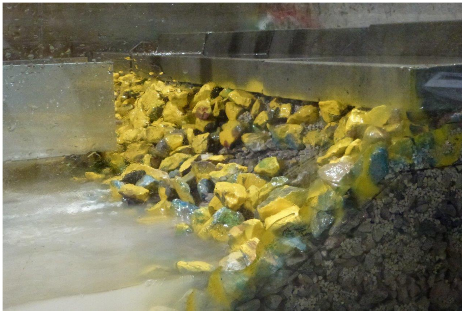
Figure 3.9: Damage to the 0.5-2 t rear side rock of a breakwater by wave overtopping.
