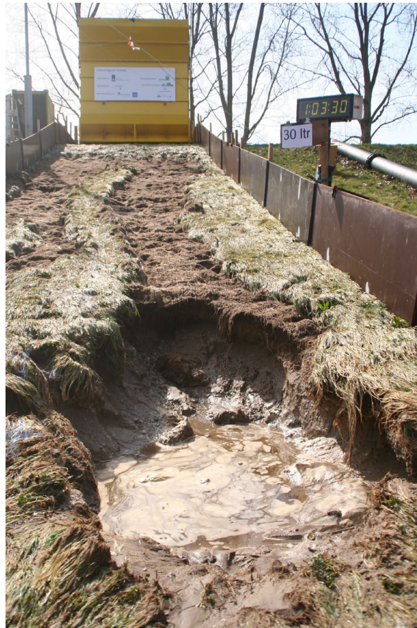
Figure 4.35 Failure of a grass covered sand dike
