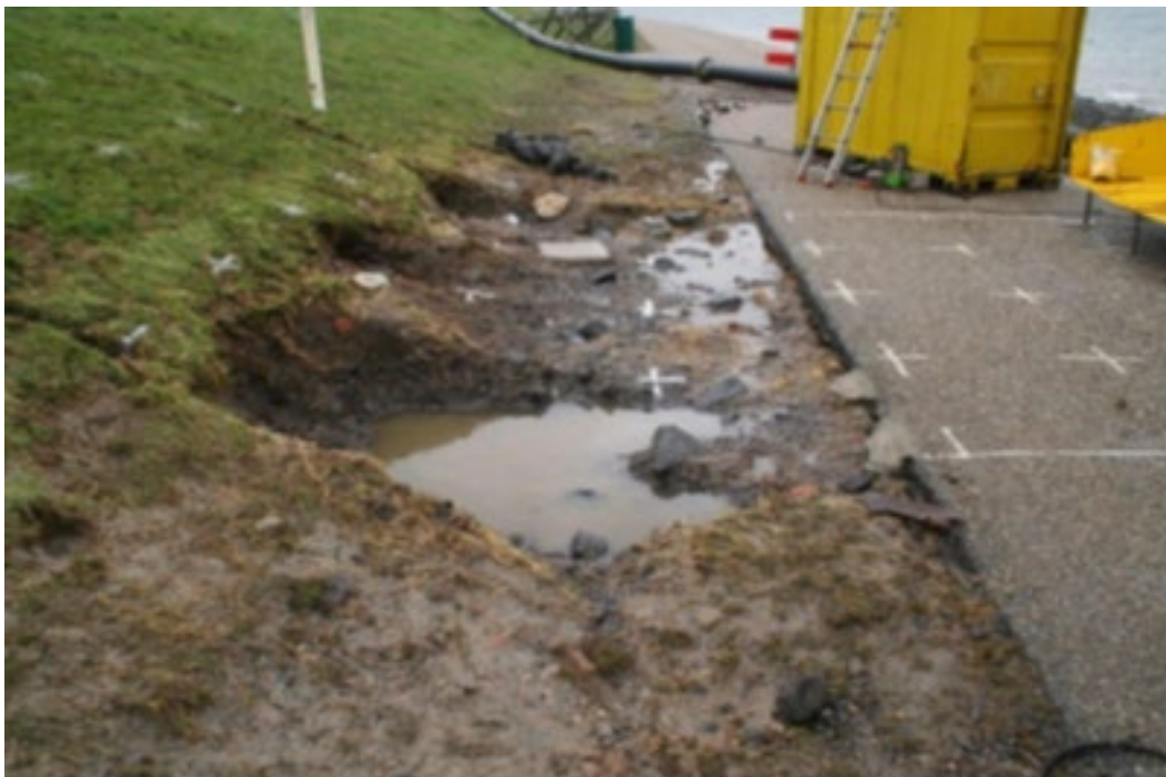
Figure 4.39 Final damage after the pilot run-up test
