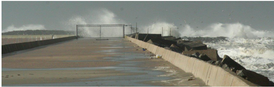
Figure 3.15 Severe wave overtopping and wave transmission at the breakwater of IJmuiden, the Netherlands
