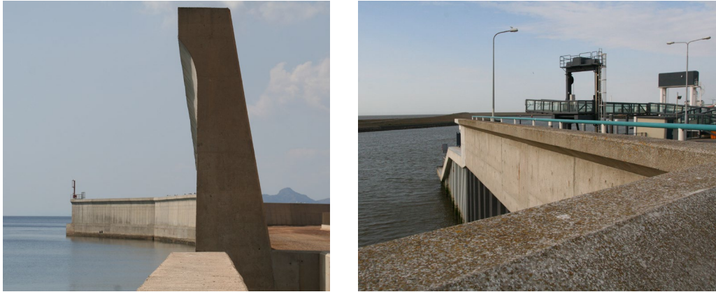
Figure 7.19: An example of a modern, large vertical breakwater with bull nose (left – Cartagena, Spain) and view on a harbour wall with bullnose under daily conditions (right – Harlingen, NL)
