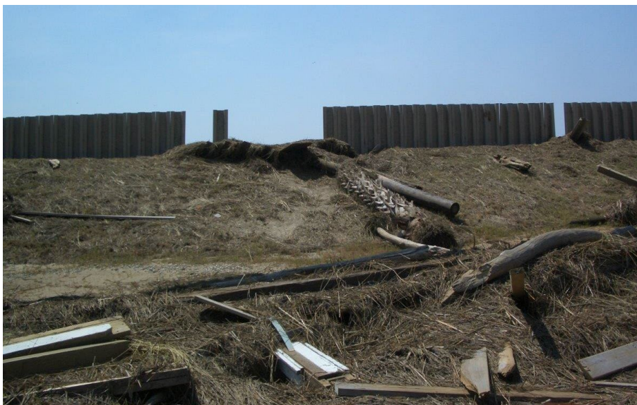
Figure 3.25: Debris such as logs in the water broke a pvc sheetpile during a hurricane and the material was transported over the crest to the landward slope. Picture taken from inside, looking at the landward slope. Gulf coast, USA
