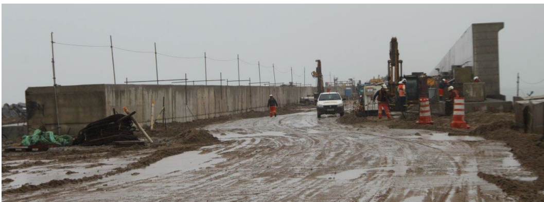
Figure 1.10: A relatively small bull nose on the crest wall of a large caisson. The caisson under construction, Açú, Brasil, is 25 m wide and the crest level is 10 m above sea level
